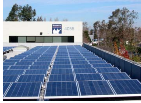
Distributed – Rooftop PV system at Swinerton, Inc. offices in Concord, CA
